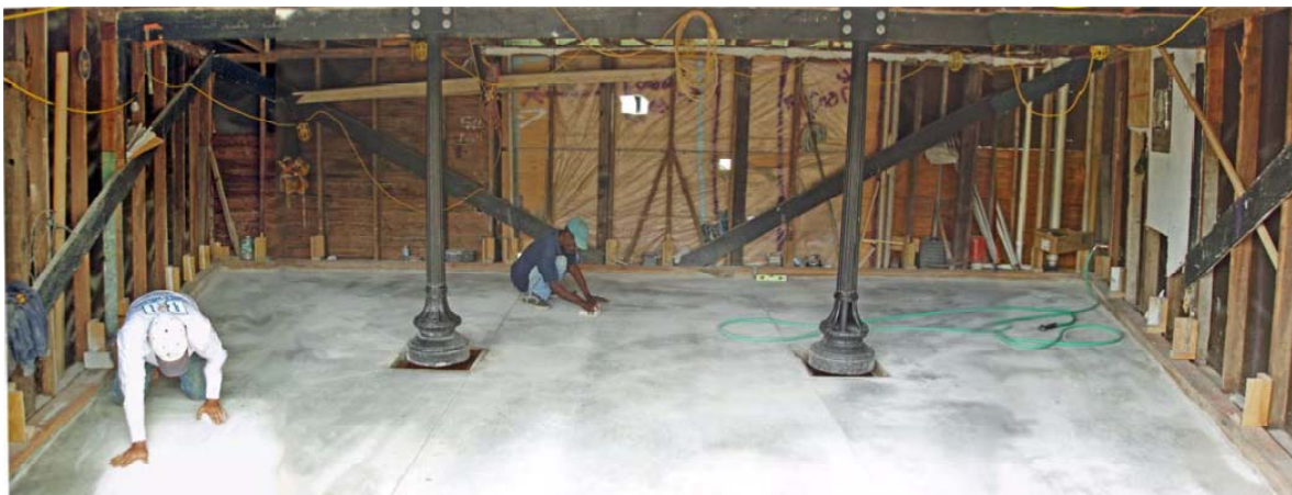
The new floor, showing the restored and reinforced lamp posts holding up the second floor. Double doors in the center of the wall will lead out to the Manor House. A single door will allow access from the catering preparation area, in the back right, to the service bar.
